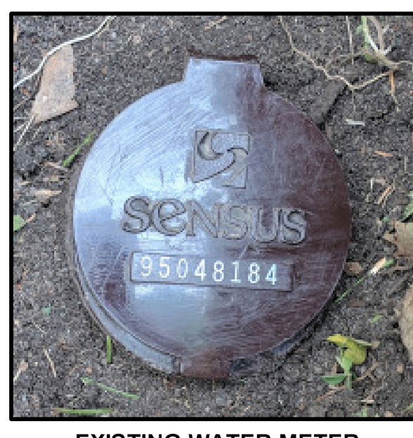
EXISTING WATER METER
